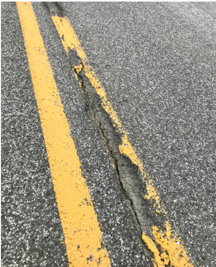
Joint deterioration before Mastic One repair
