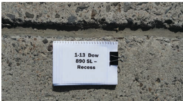
FIGURE 3 Sample of 21-year-old Dow Corning 890 SL sealant.
