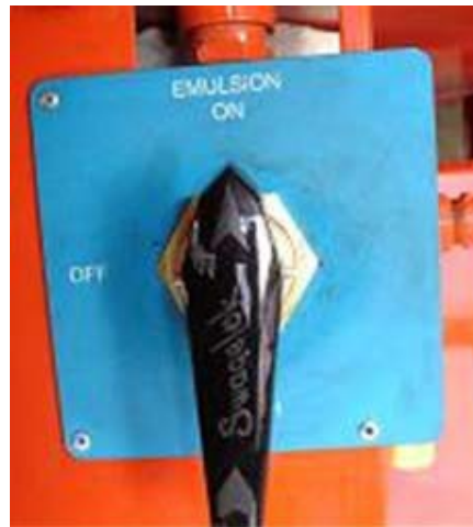
Figure 5.9 Emulsion Tank Valve
