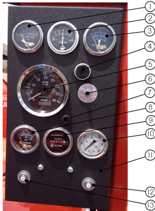
Figure 9.22 Engine Control Panel
