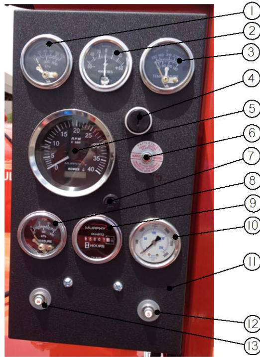
Figure 9.22 Engine Control Panel
