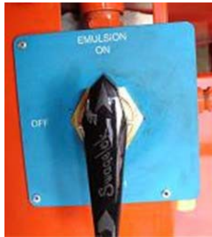
Figure 5.9 Emulsion Tank Valve
