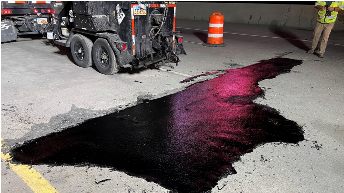
Second and final lift of Mastic One was installed added structure and stability back into the distress. The flowable characteristics provide smooth transition and improved safe driving experience.
