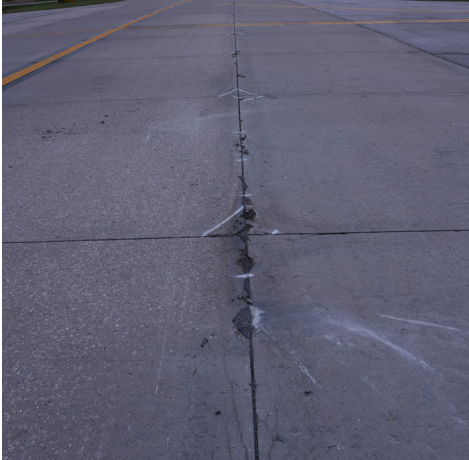
Deterioration on taxiway prior to repair.
