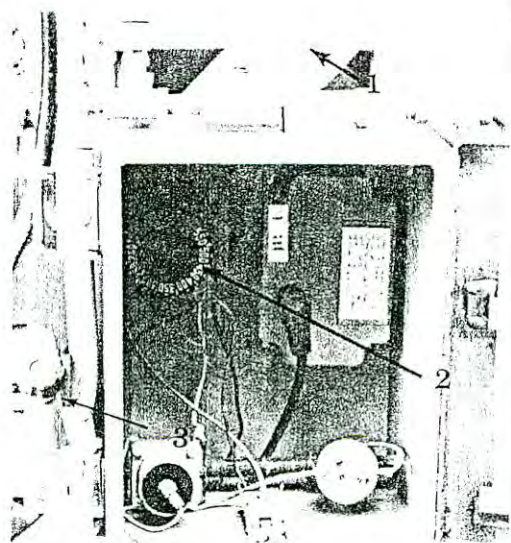
FIGURE 7 — Automatic Burner Control
