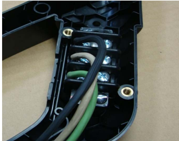
Figure 6.17 Terminal Block Wiring
